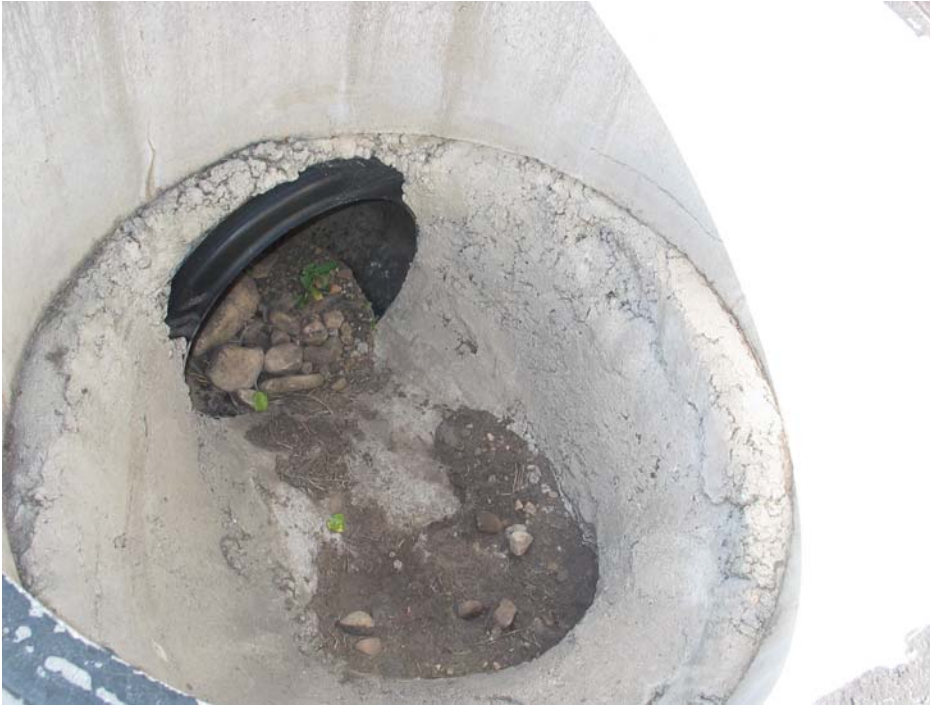
View into inside of culvert – estimated to be less than 34 inches high
